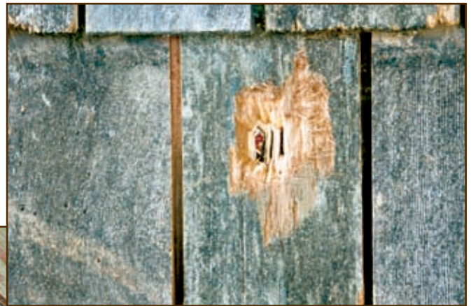
Photo 3C – Actual pressure-washing damage. This type of damage is typically caused by inexperienced equipment users. Contact CSSB for care and maintenance of cedar shingles and shakes.
